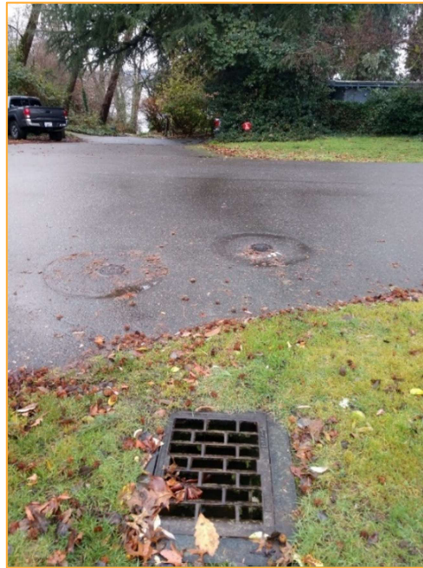
Photo S11 – Facing west along the north side of SE 30 th St approximately 130 feet west of Photo S10 at the northeast corner of the intersection of SE 30 th St and 60 th Ave SE. Runoff is conveyed west toward Lake Washington.
