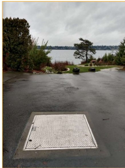
Photo N10 – Facing west in Calkins Landing approximately 95 feet west of Photo N9. Runoff is collected in the pre-settling vault pictured before being discharged into Lake Washington.
