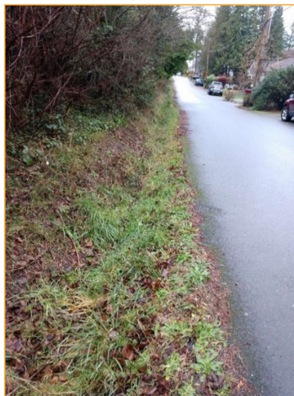
Photo S4 – Facing south on the east side of 62 nd Ave SE approximately 60 feet from Photo N4. Onsite runoff sheet flows in the southwest direction toward the ditch above and is conveyed south to be combined with the south basin downstream conveyance system.
