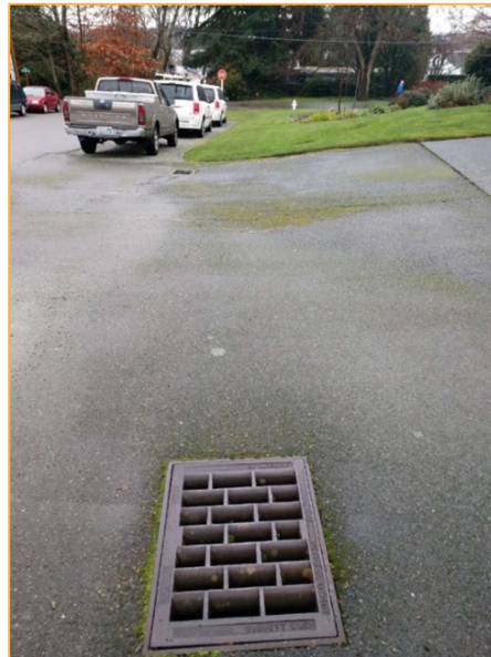
Photo S10 – Facing west along the north side of SE 30 th St approximately 30 feet west of Photo S9. Runoff is conveyed west toward Lake Washington.
